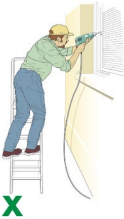
Incorrect Steps side-on to work activity.
